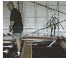
Mr. Kermit Severson, Installation Supervisor of Rohn Products Phils. assembles the Jampro JHPC-8 Antenna
